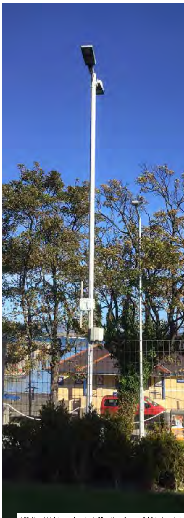
LED Street Light also showing Wifi unit on Queens Rd Dún Laoghaire
