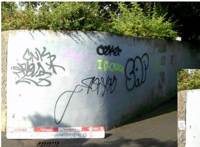
Graffiti Removal in the County – before...
