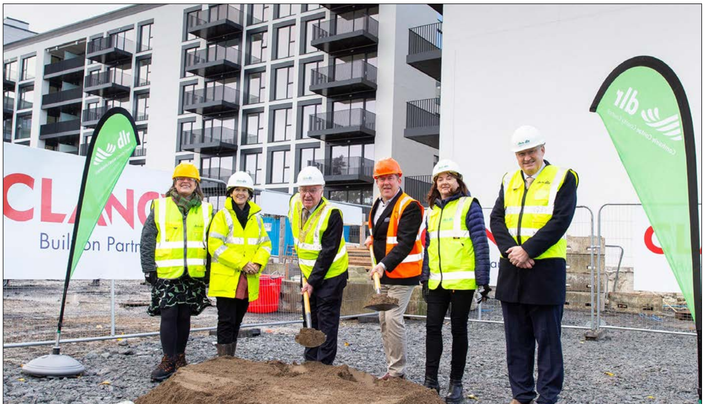
St. Laurence's – Turning of the Sod at St. Laurence's – 88 new homes under construction
