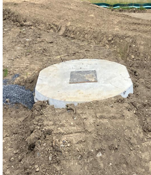
Septic Tank at Compound Location
