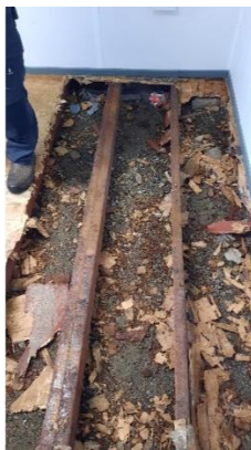
Rotten floor of old unit
