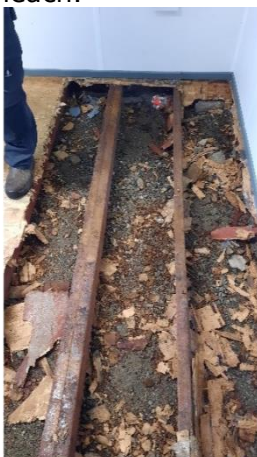
Rotten floor of old unit
