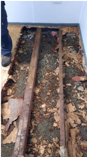
Rotten floor of old unit
