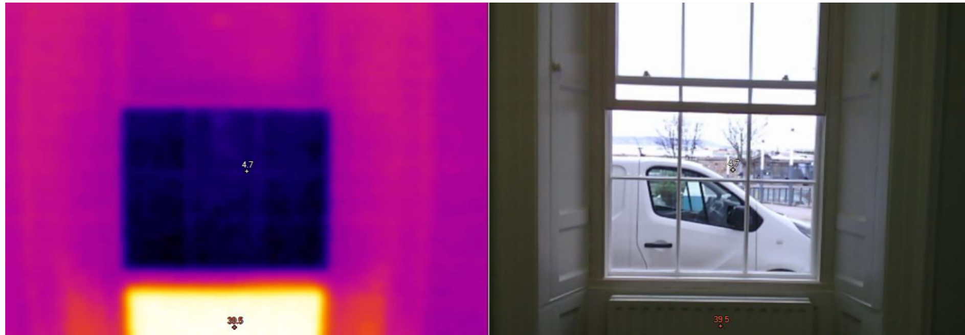
Figure 28 Thermal image with secondary glazing open
