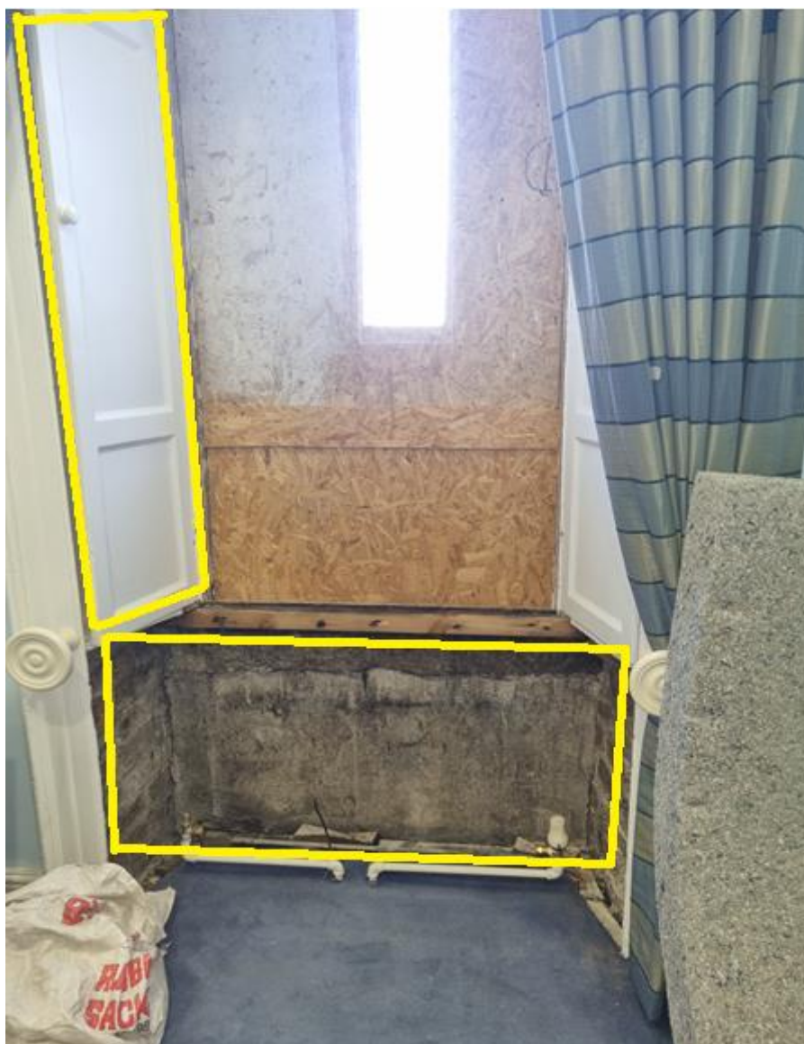
Figure 9 Void behind radiator exposed & behind shutter box marked in yellow
