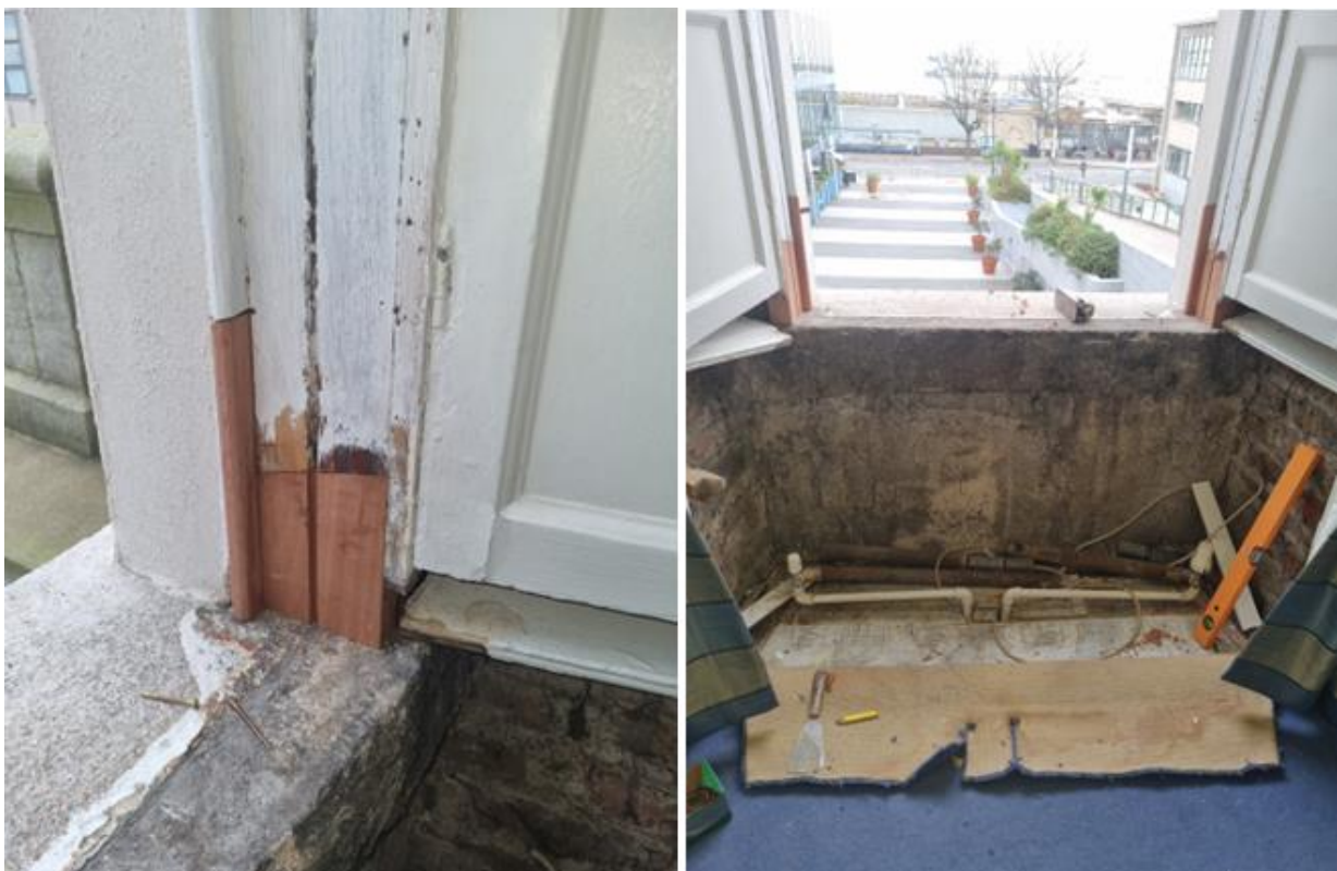
Figure 10 Bottoms of all window frames rotting and repaired with Mahogany
