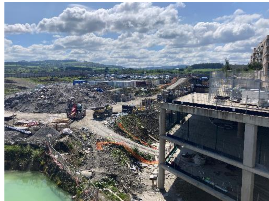
TCC1A looking towards TCC1B and TCC3, showing the existing podium and basement levels. Huge cost in this construction with complicated occupancy characteristics
