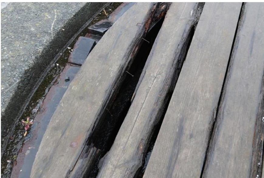
Plate 40: Rot in boards on the turntable platform
