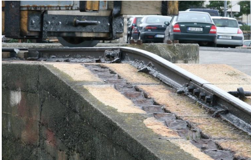
Plate 51: Bend in rail at break in slope
