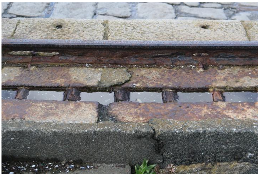
Plate 52: Rack alongside track
