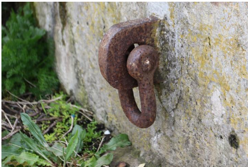
Plate 44: Shackle below bearing on western side of turntable
