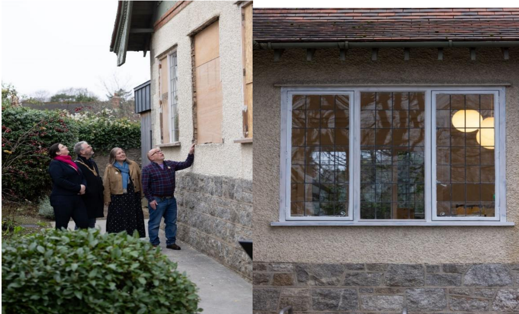
Before and after – ongoing conservation works to Cabinteely Library windows (Credit: Coalesce)
