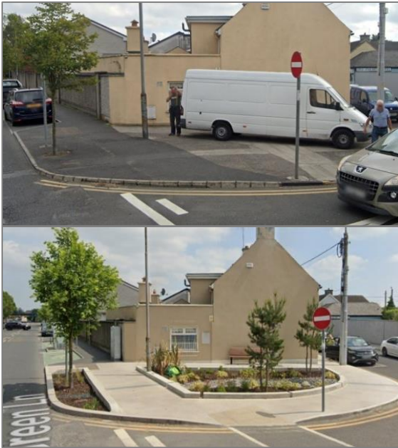
Figure 15-5: Before and After the installation of a Rain Garden at Green Lane / Pollerton Road, Carlow.
