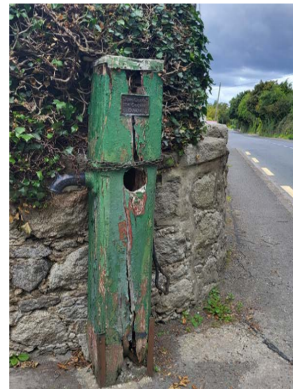
Wooden exterior standing water pump on Enniskerry Road
